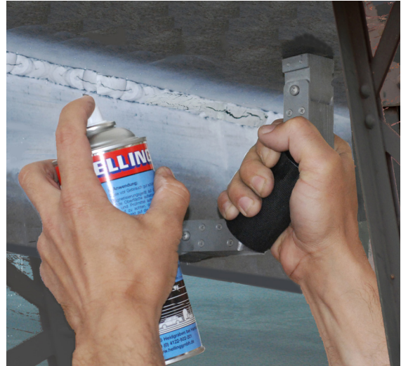
Weld joint inspection on a bridge by use of BW 333 black magnetic particle suspension and NR 104 A white background paint.
